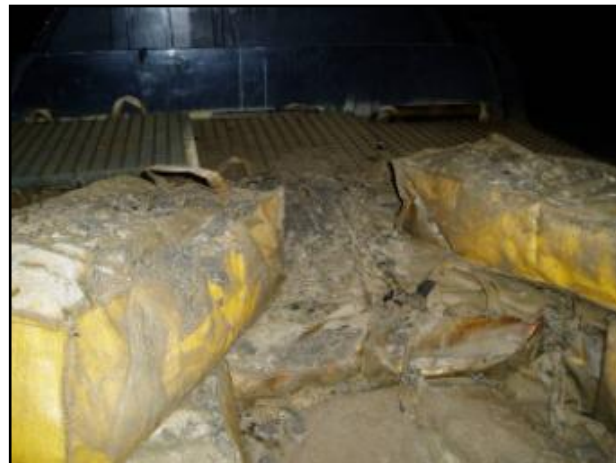
Figure 2. Perlite filter media needs replacement.
