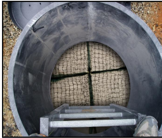
AF-3.48 ingress/egress ladder and wedge-shaped filter containers. Cargo netting also shown.
